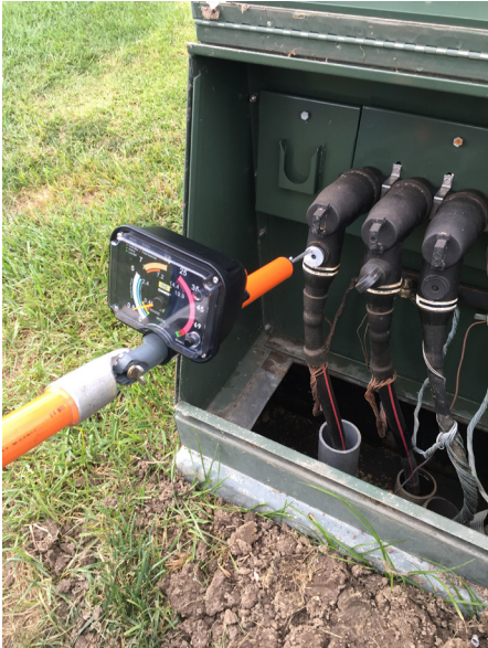
Testing a Capacitive Test Point on dead-front elbow
