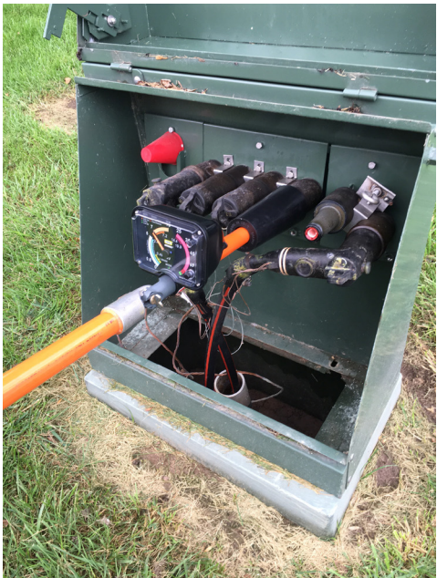
Taking a reading with the MRVI with Bushing Adapter on dead-front equipment
